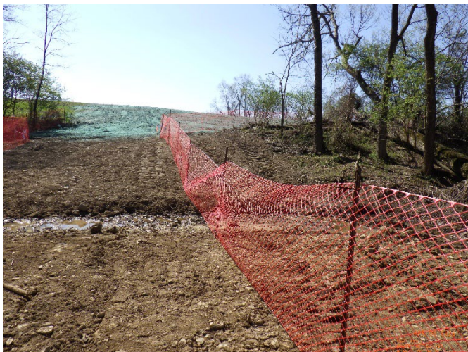
5. Stream crossing area not protected with temporary E&S BMPs.
