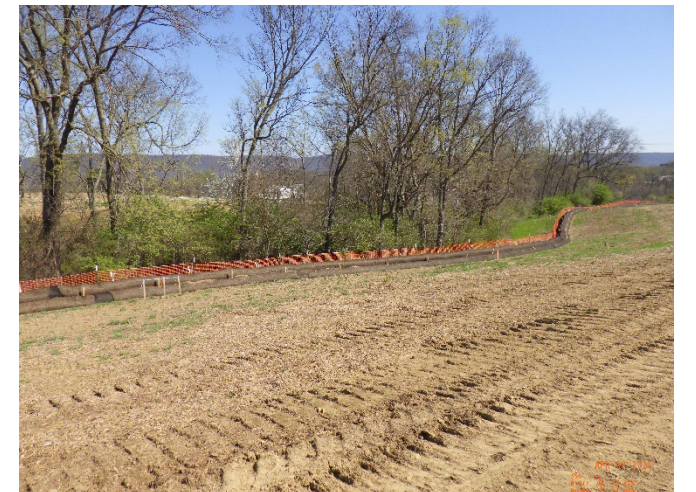
6. Stakes on filter sock sediment traps not tied with wire.
