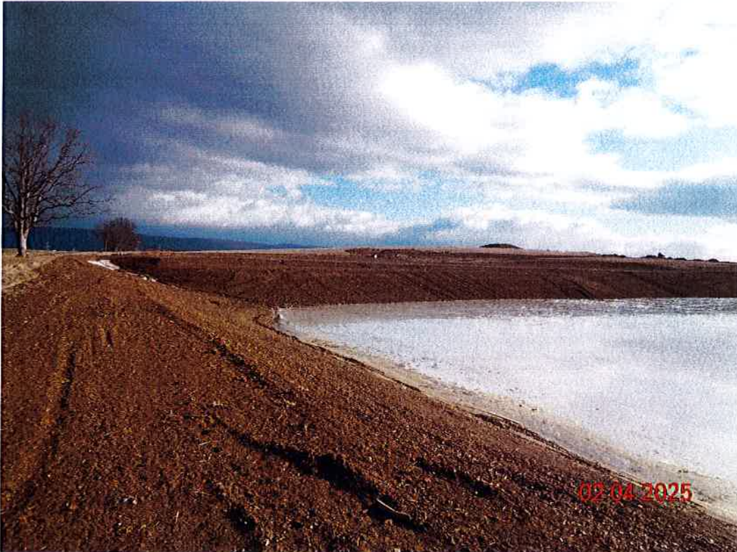
1. Sediment Basin A not installed per plans. Temporary baffle not installed.
