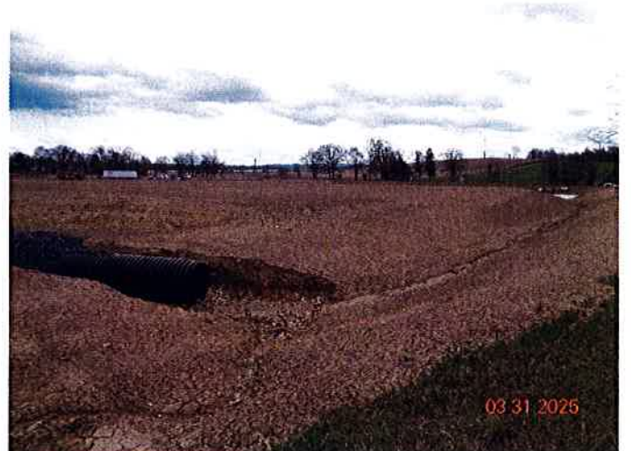
6. Swale 14 not topsoiled, seeded, mulched, and matted.
