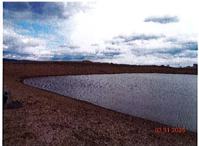
2. Temporary baffle not installed in Sediment Basin A.
