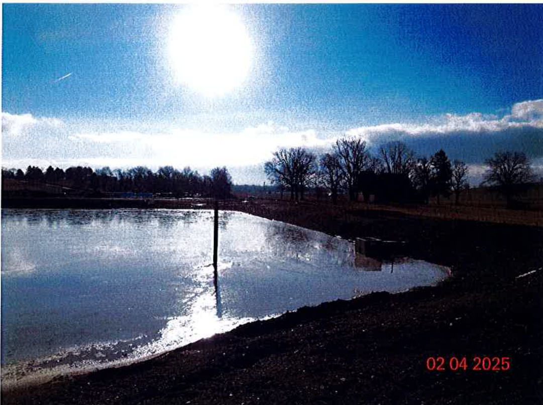
2. Sediment Basin A not installed per plans. Riprap apron, trash rack, and skimmer not installed.
