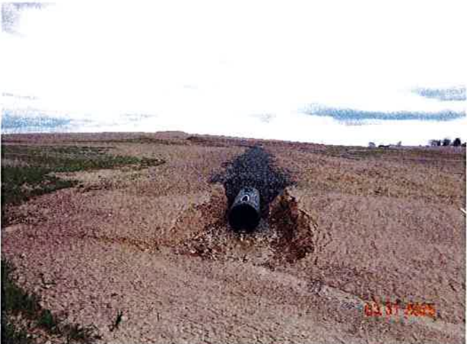
5. Riprap apron M not installed.
