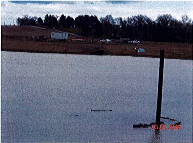
3. Riprap apron G3 and flared end section not installed in Sediment Basin A.
