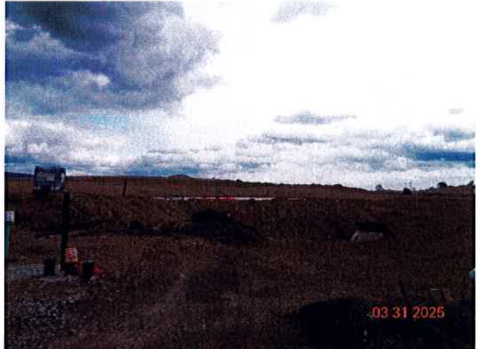
4. Pipe outlet from Sediment Basin A and riprap apron G not installed.
