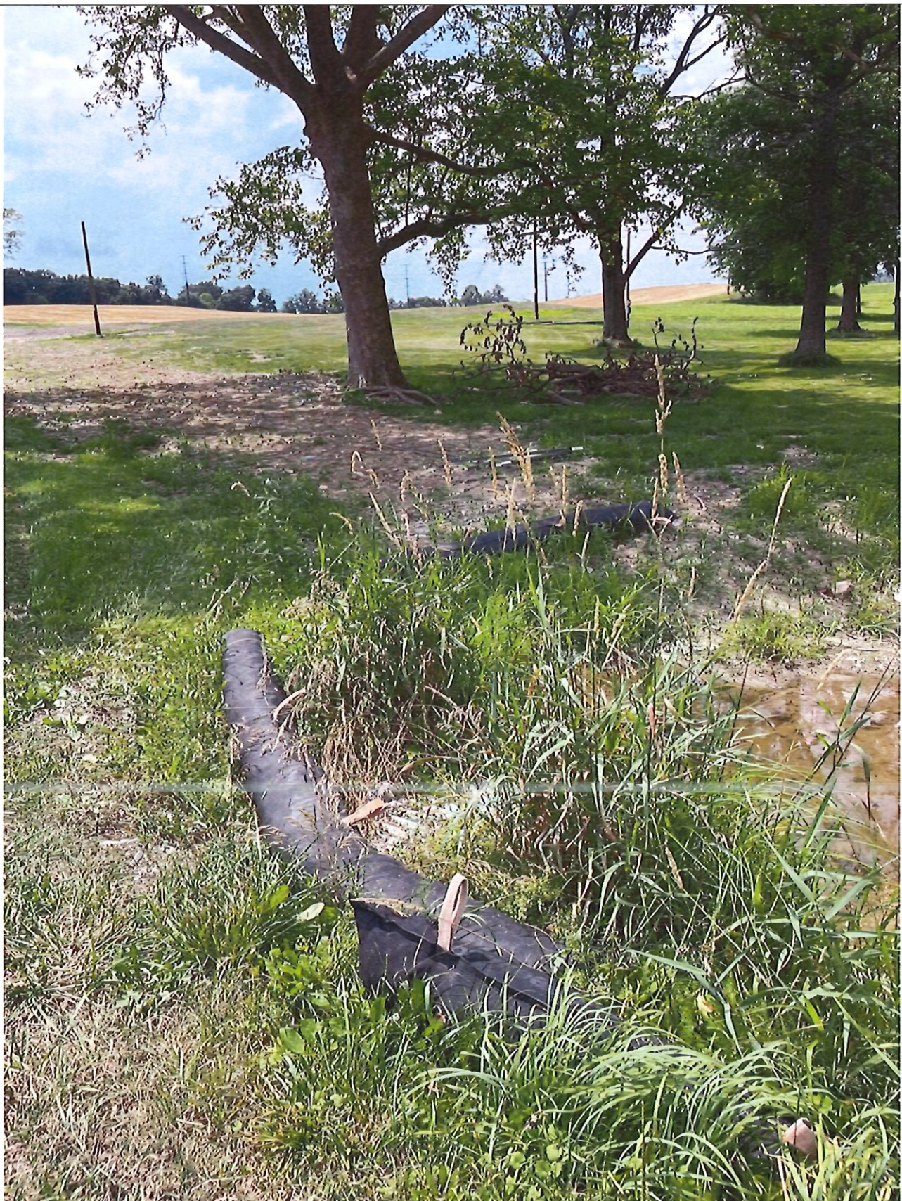
Photograph depicts impacts to Wetland C/Channel1 per the wetland delineation report for the Bolt Project as a result of the Cumberland Knoll Phase 1 Forced Main installation.
